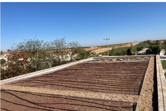
Figure 3 Implementation of the irrigation system.
