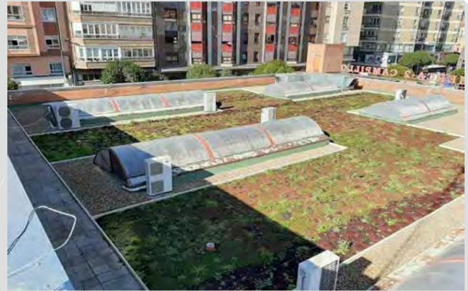
Figure 6. Green roof in the municipal market of El Campillo in Valladolid (Source: Valladolid City Hall).
